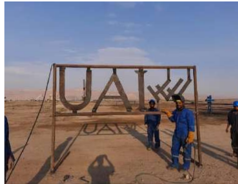
Manufacturing of Metal Structures
